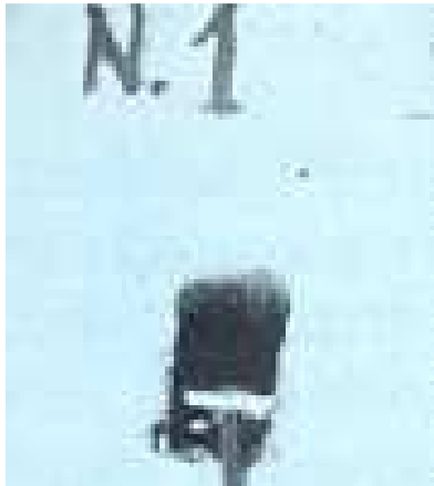
Cable is open to inspection and SINIT tee is placed to inject resin.
