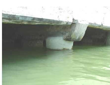
View of the rehabilitation with Subcom T.260 replacing concrete between piles and platform
